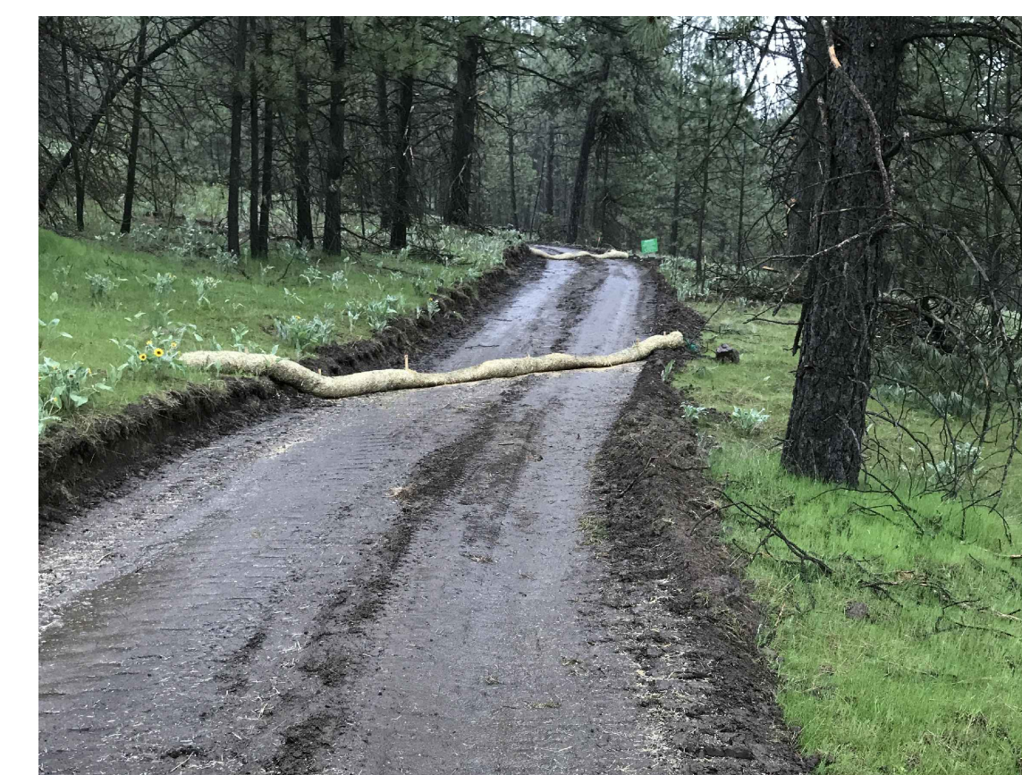
7. MINOR ROAD CUT/FILL
